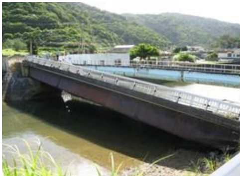
A collapsed bridge by aging
