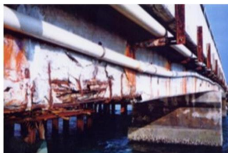
Corrosion condition of sea bridge
